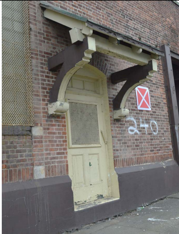
242 Spruce Street (Presently referred to as 240 Spruce St.) – detail of west side entrance
