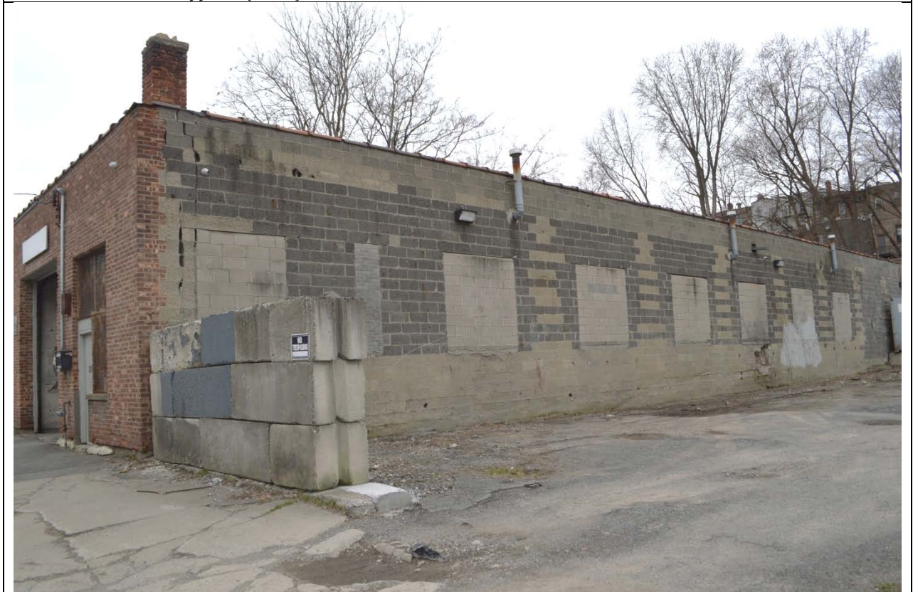
216 Elk Street – view of side (west) elevation.
