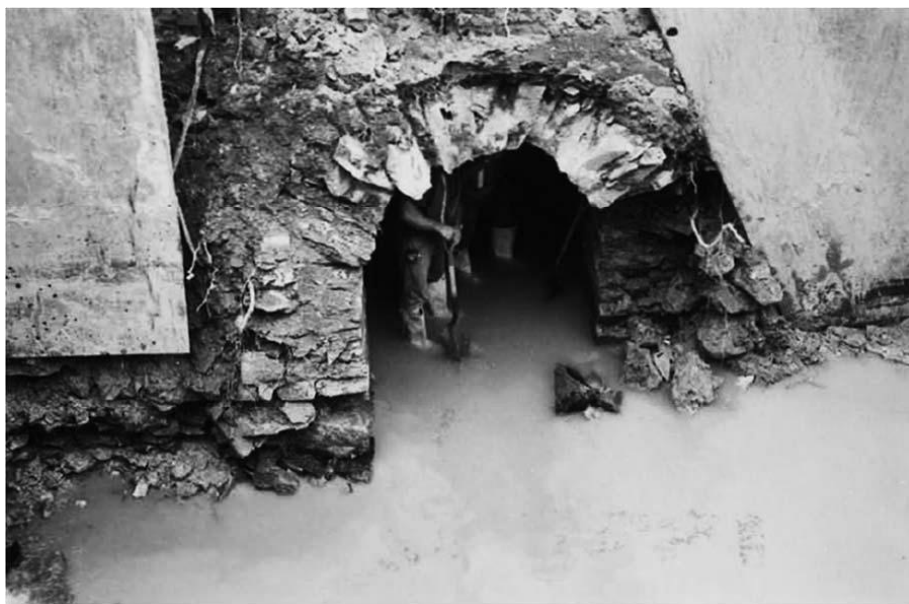
Figure 3. Early to mid-19th-century Fox Creek culvert at North Pearl Street. View west.
