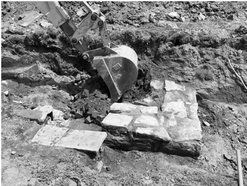
Photo 17. Removing the demolition fill inside of the southeast corner of 238 Clinton Avenue. View northeast.
