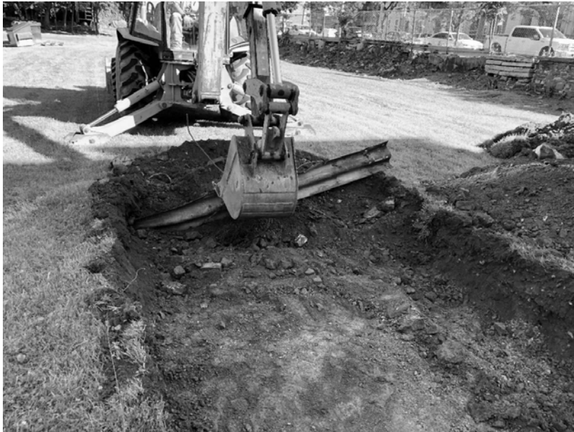
Photo 28. Removing the first of ten guardrails buried in modern fill of Trench 4. View northwest.
