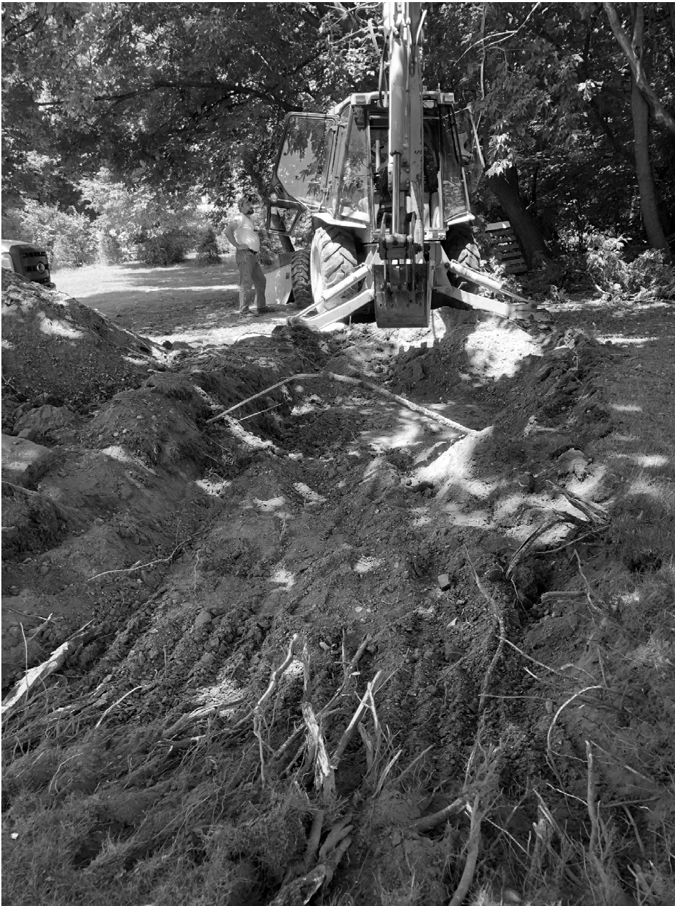
Photo 27. Trench 6 which was abandoned after the backhoe had a mechanical failure preventing additional excavation. Exposed pipe in the middle was a steel pipe with two copper lines inside. It was determined that it was not an active utility. View northeast.
