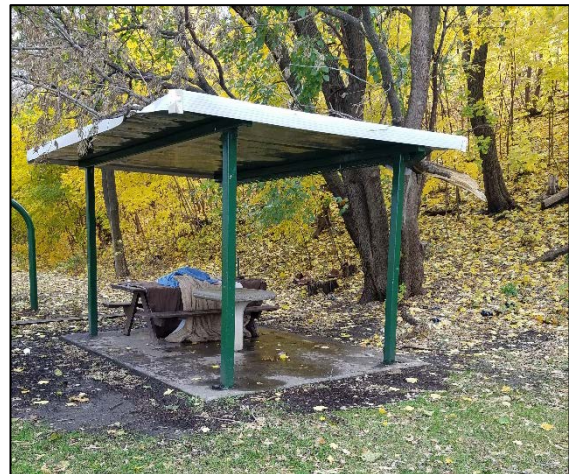
Figure 19. Sheridan Park Pavilion-Stormwater Runoff Photo by TJ Kennedy
